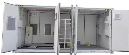
1075KW HH ESS
