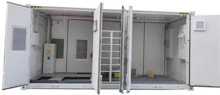
1075KW HH ESS
