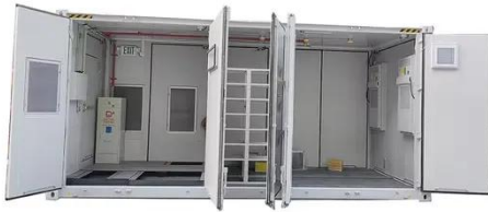
1075KW HH ESS
